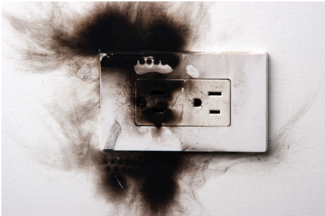
Scorch marks on cover plate
