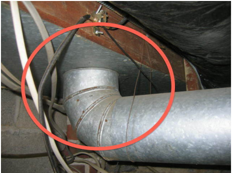
Loose connection; recommend sealing.
