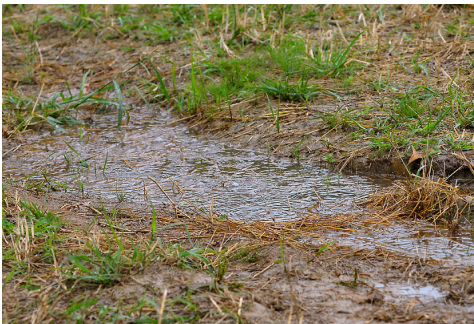
Water pooling in yard; recommend drainage
